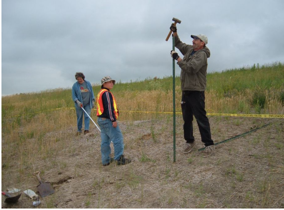
Here is Jack Bauer starting the fencing. The dig area has to be fenced in to protect trespassers, human and others.
